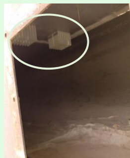
Figure 14: Heat sink inside the boiler
