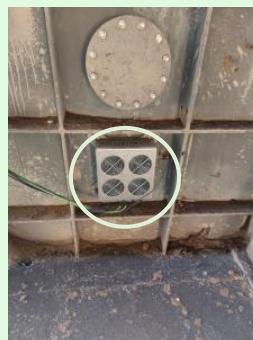
Figure 17: installed WHRU system
